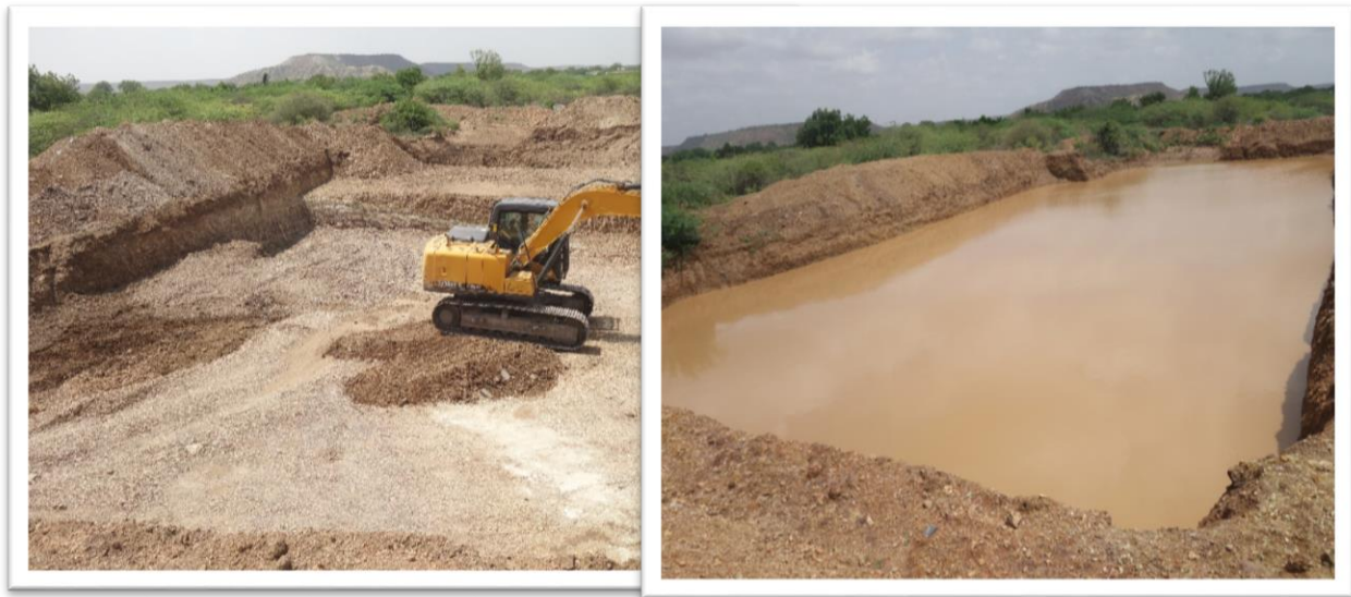
Figure 19. Percolation tank created on a stream in the watershed – before and after rain.
