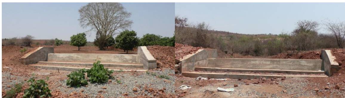
Figure 2. Check dams constructed in Kurnool watershed in (L) Repalli village and (R) Venkatagiri.
