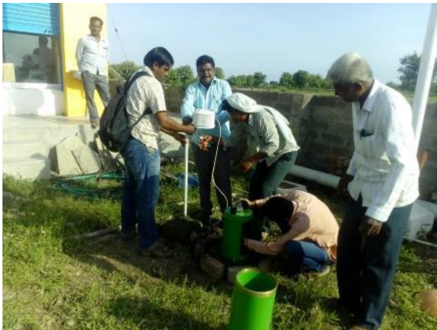
Figure 10. Dual type automatic-cum-manual rain gauge installed in Ukkali watershed.
