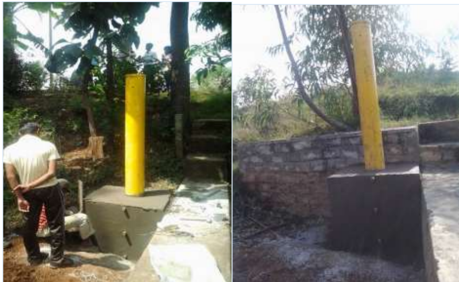
Figure 34. Hydrological monitoring station installed at Chikkamagaluru.
