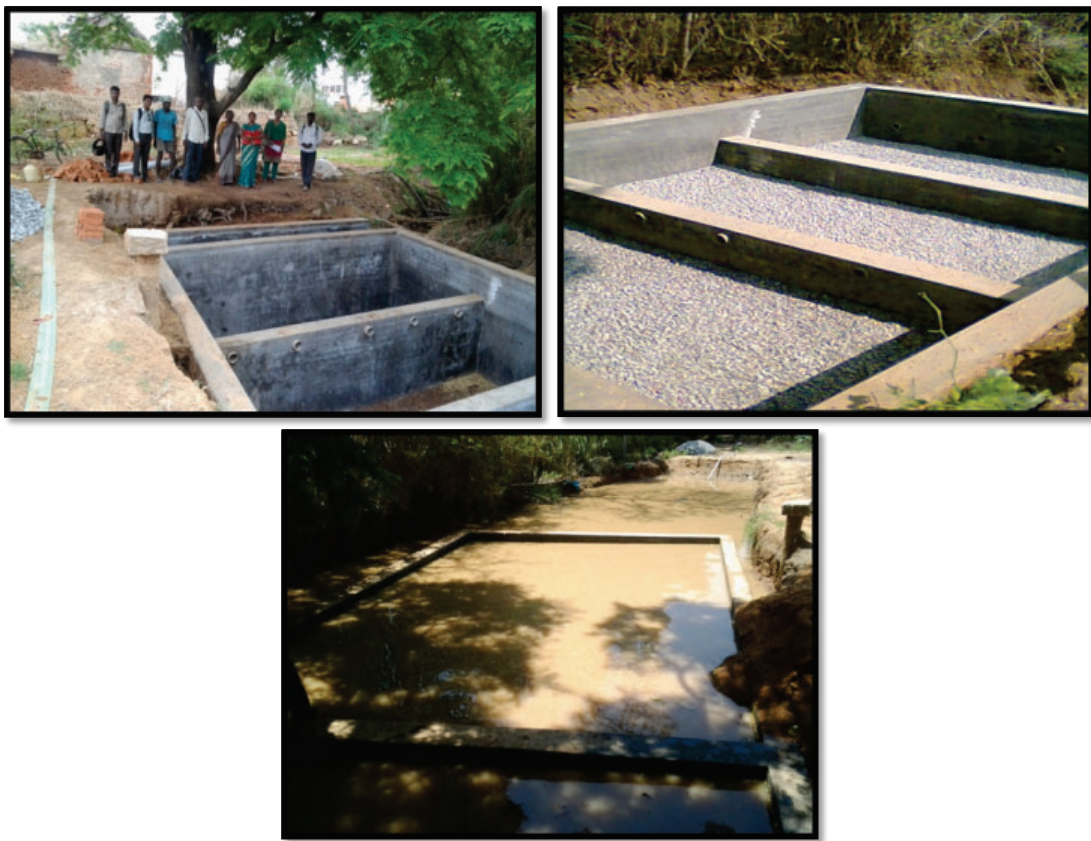
Figure 10. Constructed wetland for domestic wastewater treatment in Mudavatti village, Kolar
